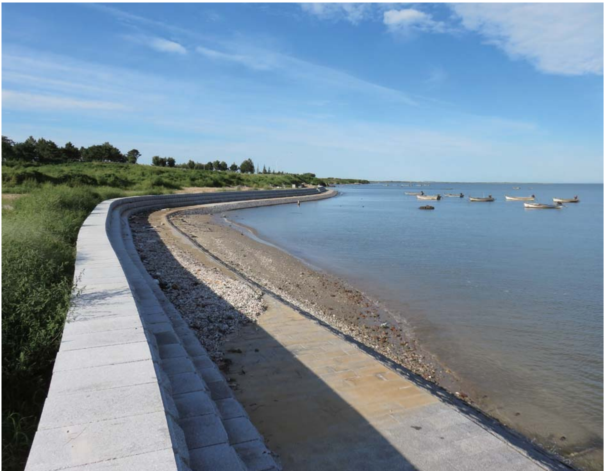
The comprehensive improvement project phase I of the north coast of Sanggou Bay supported by Rongcheng Branch
