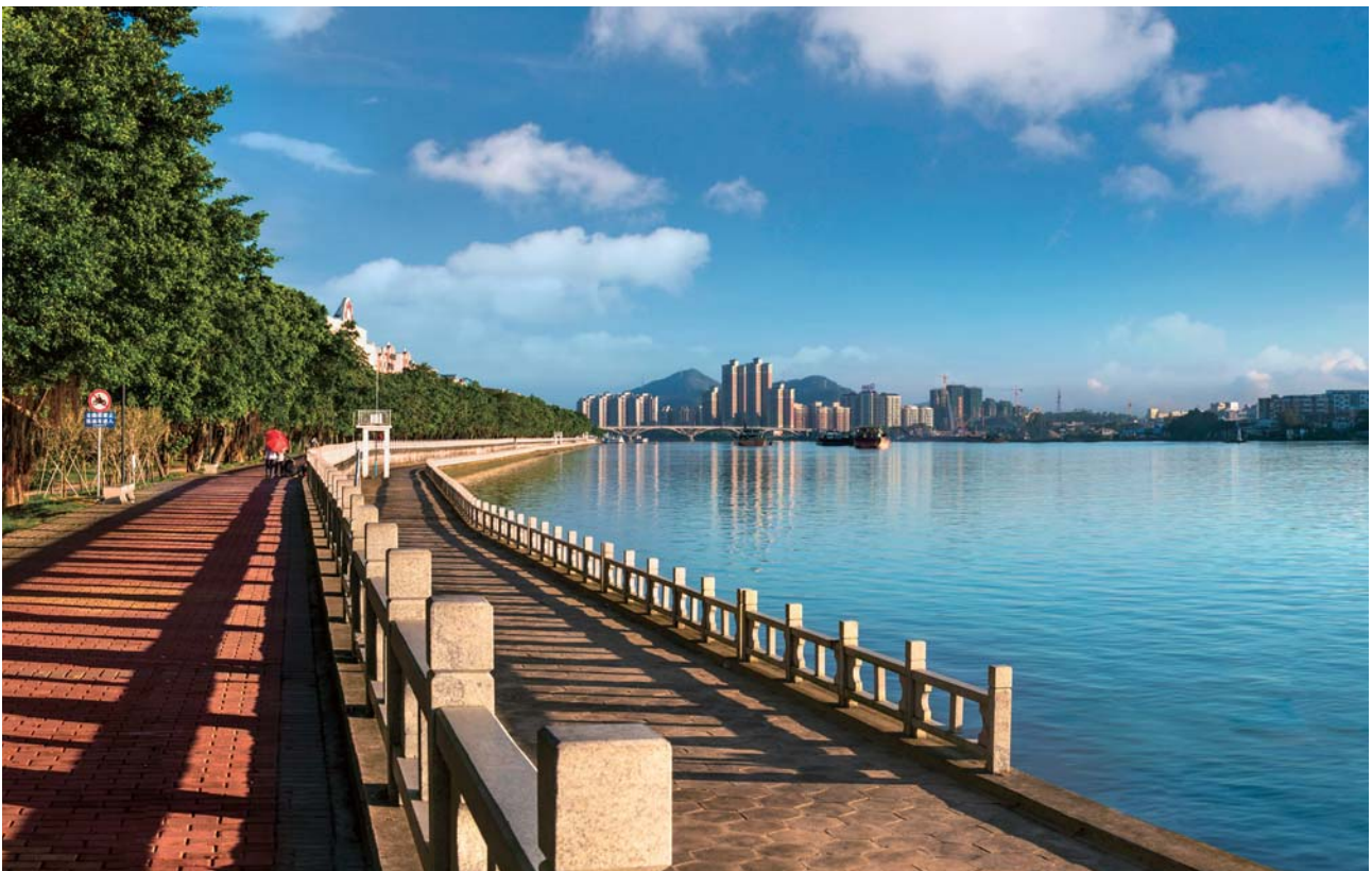
Support for Construction of Zhuhai Doumen Jing'an Town Floodwall Reinforcement Project by Zhuhai Branch
