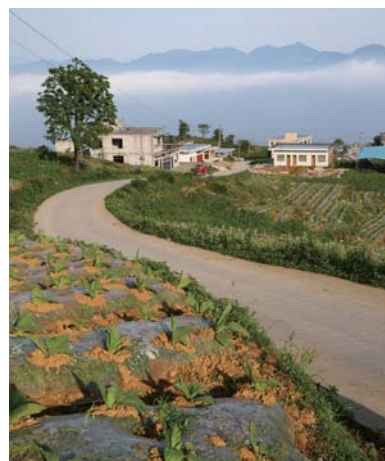
Construction project of rural roads in Bijie City of Guizhou supported by ADBC
